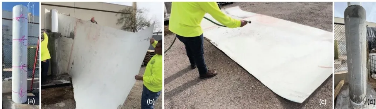
Fig. 3. Field application: (a) FLF placed and filled with concrete, (b) removing the laminate after concrete hardens, (c) cleaning and saving the laminate for future use, and (d) smooth concrete finish with no spiral marks
